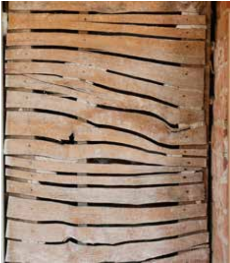
Historical accordion lath revealed during interior restoration. This form of hand-split wooden lath was commonly used for plastering walls until about the mid-19th century.
