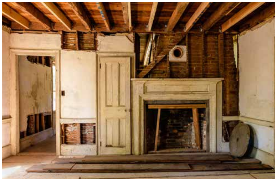
Restoration underway at the rear parlor/dining room interior, 2018 (Photo by William P. Steele, courtesy of the Yaphank Historical Society, detail).
