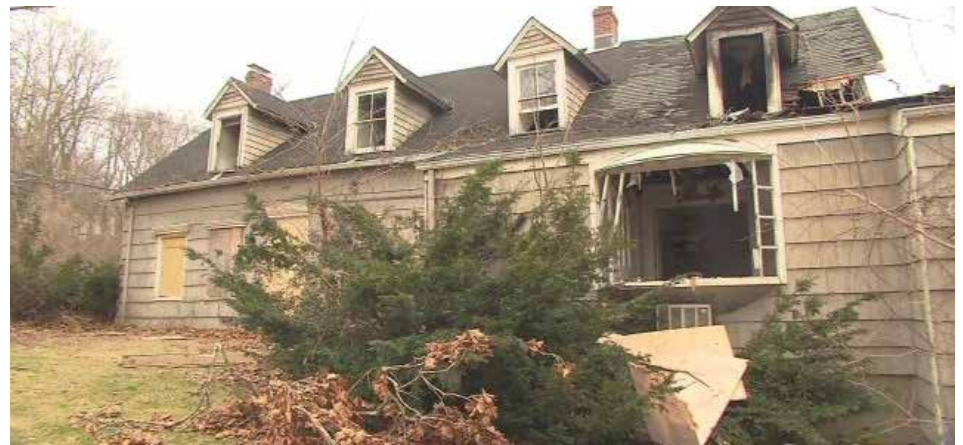
Fire damage in the Mill Pond House was mostly concentrated to the twentieth century additions.
