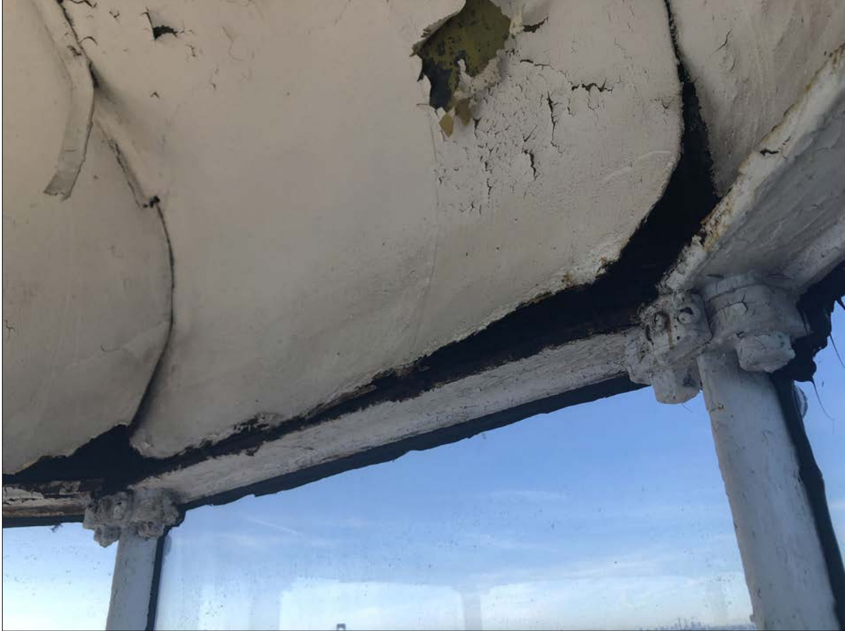
Photo 11. Breaches in Lantern dome liner. The nature of the damage seems to indicate vandalism rather than the result of natural effects, such as rust jacking or ice forming behind the sheets. Inner surfaces are very wet.
