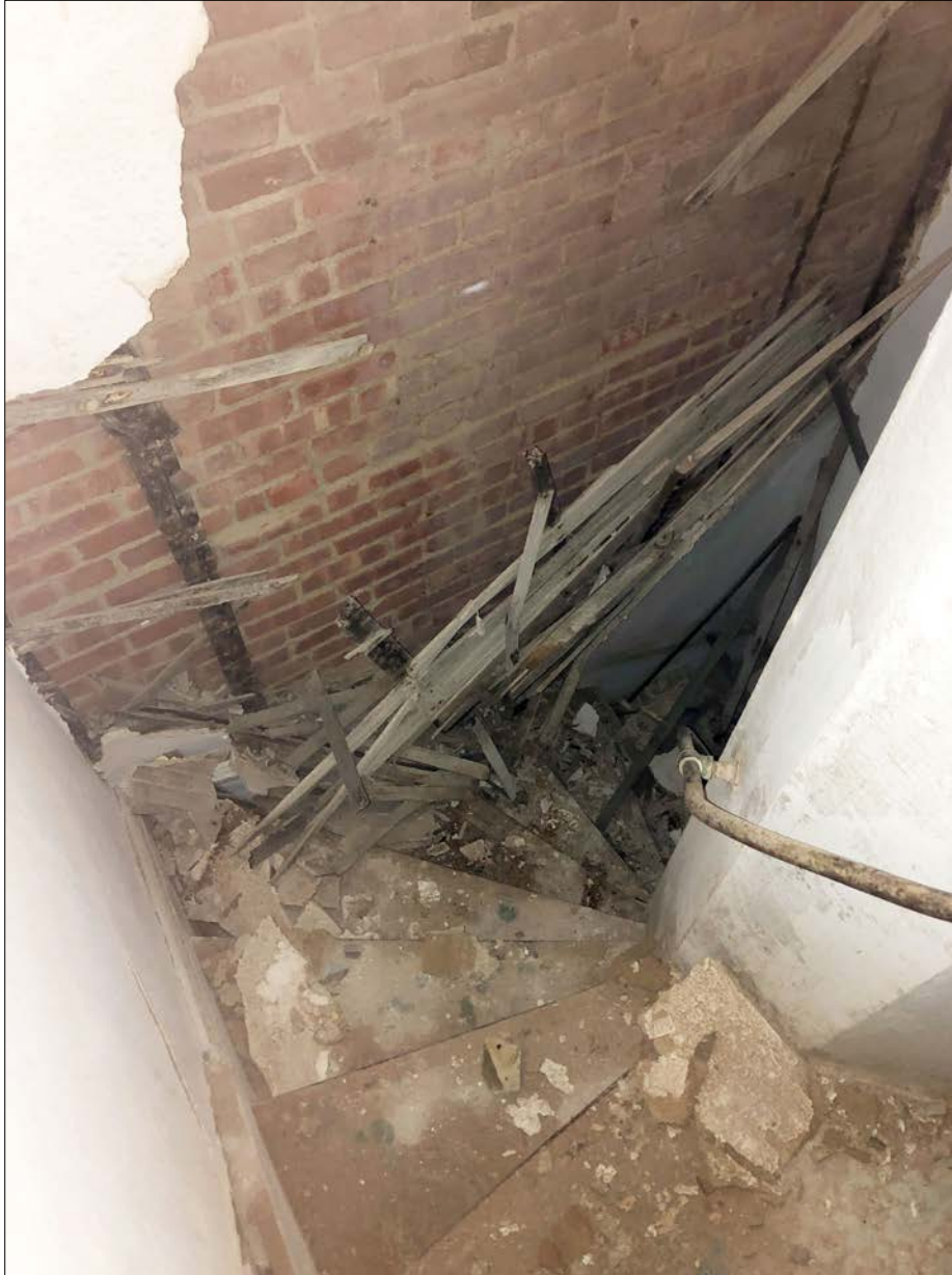
Photo 7. Collapsed plaster & lath of the Tower stair, looking down. This is the direct result of water entering the structure and rusting the lath nails, and is a surface condition, not a structural failure. The Tower's dislodged masonry must be addressed (Photo 8) to stabilize this condition.
