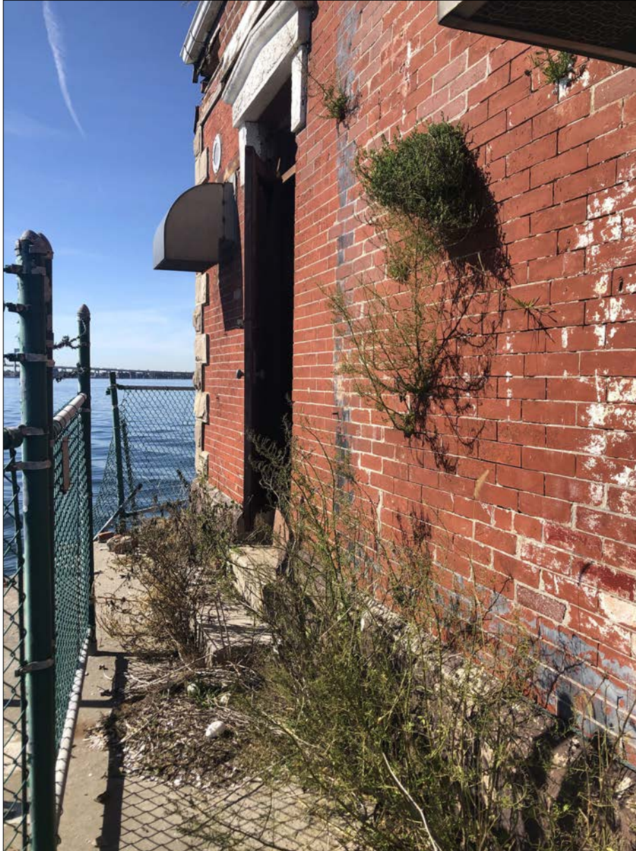
Photo 4. View of south (landing) facade and unsecured entrance door, looking W. Nesting, vegetation and generally unkempt conditions send a signal that the site has been abandoned, which invites unauthorized access. Evidence of this already exists, and may affect the USCG's ability to properly maintain the light, which is an active aid to navigation.
