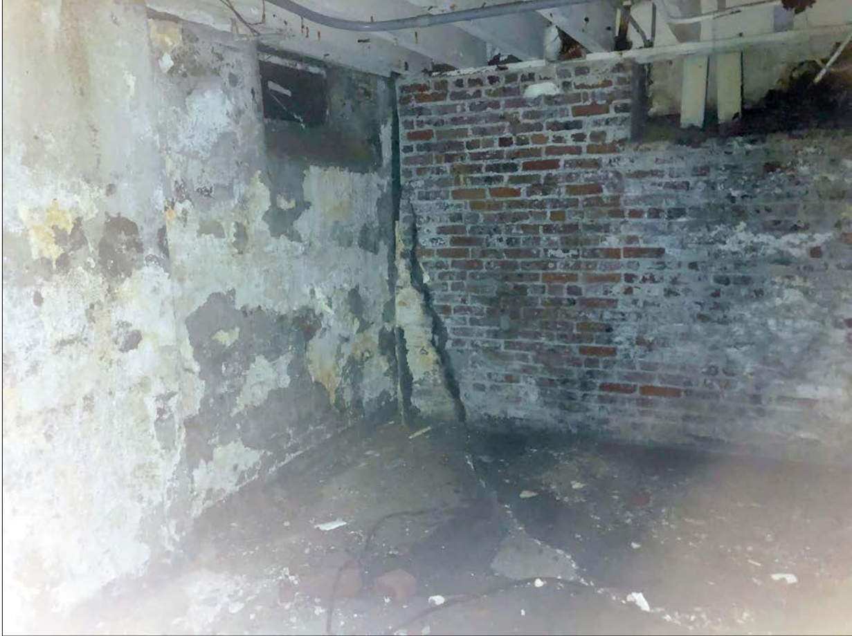
Photo 5. Propagation of a crack through the concrete and masonry foundation was noted in WSA's 2017 condition survey. The crack continues to open because of the effects of ice forming, but it is not affecting adjacent elements significantly more than already noted in 2017.
