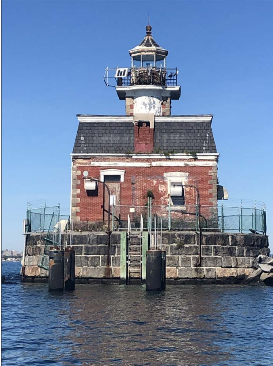
Photo 2. View of Stepping Stones Lighthouse, looking north. Surface conditions have worsened since WSA's 2017 report, but the underlying structure remains sound and imminently restorable. For now, stabilization of the site is paramount.
