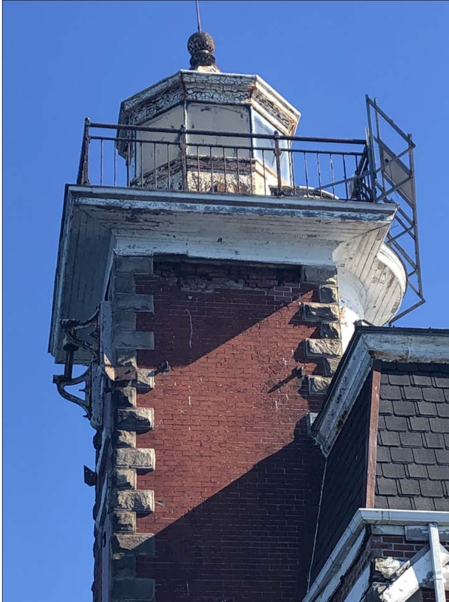
Photo 8. Dislodged brick at the upper reaches of the Tower's west facade was noted as a high priority concern in WSA's 2017 condition report, yet was never addressed. It has gotten worse, including fallen granite blocks in addition to the brick masonry. Resulting breach is unstable long-term, and allowing water to enter the Tower interior stairs, causing further damage. If attended to, this is a very straightforward masonry repair; if ignored, it's negative effects will accelerate.
