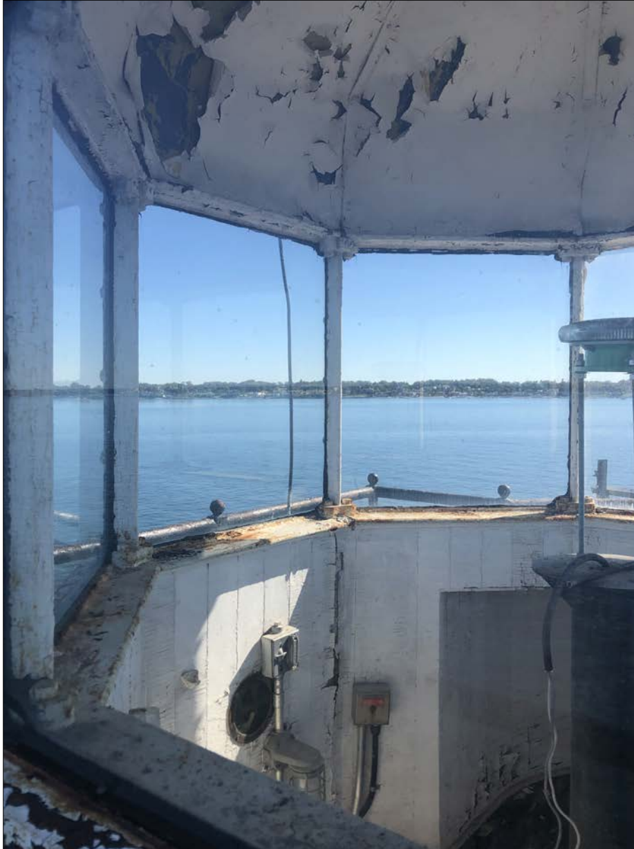
Photo 10. View of Lantern looking SE, toward King's Point. Generally, the space and its features are in relatively stable weathertight condition, with the exception of the dome liner, which shows damage likely related to unauthorized access via the unsecured south entrance door.
