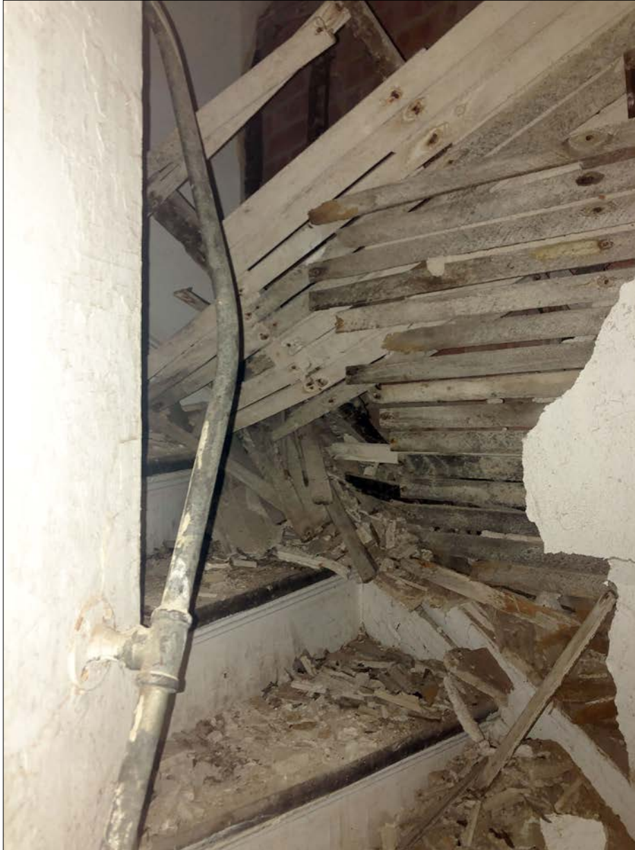
Photo 6. Collapsed plaster & lath of the Tower stair, looking up. This is the direct result of water entering the structure and rusting the lath nails, and is a surface condition, not a structural failure. The Tower's dislodged masonry must be addressed (Photo 8) to stabilize this condition.
