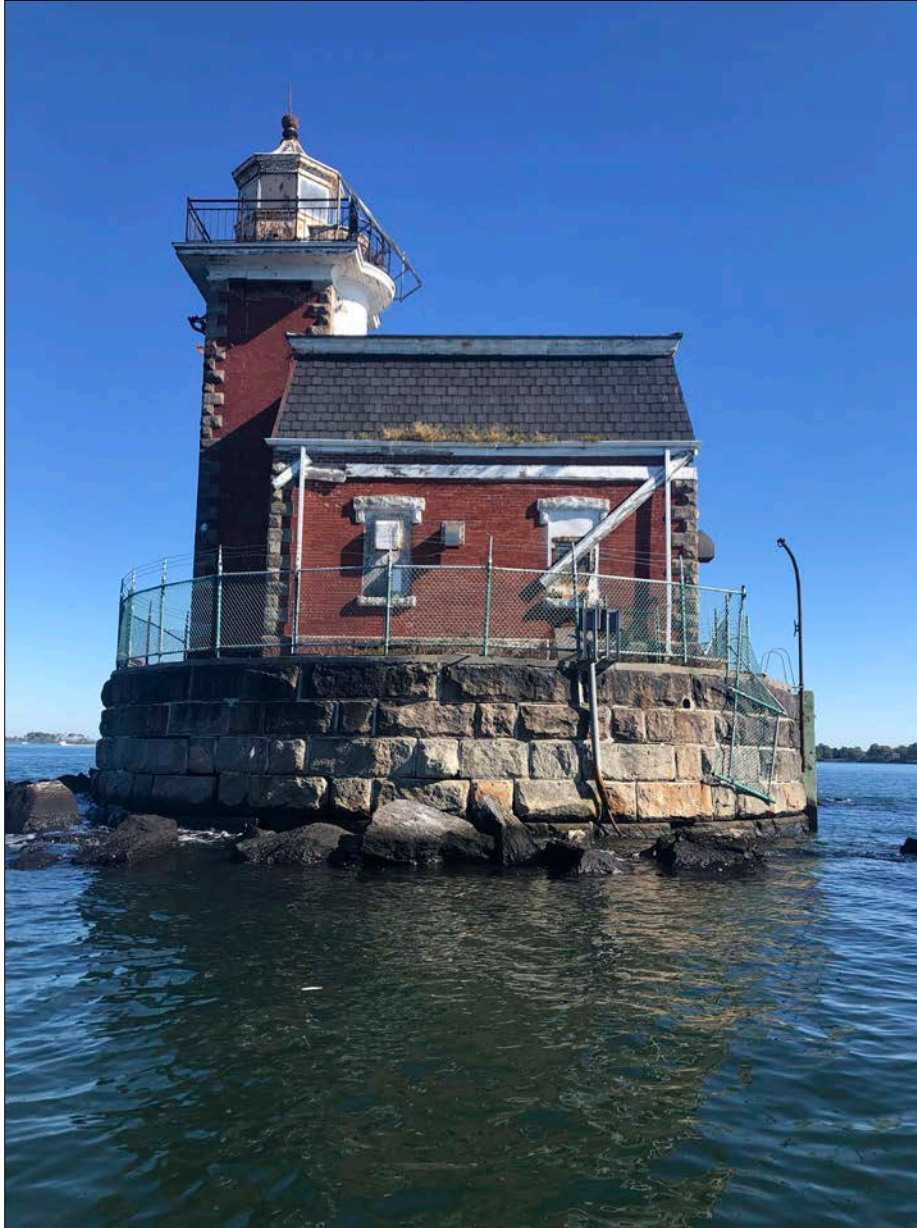
Photo 3. View of Stepping Stones Lighthouse, looking east. Surface conditions have worsened since WSA's 2017 report, but the underlying structure remains sound and imminently restorable. For now, stabilization of the site is paramount.
