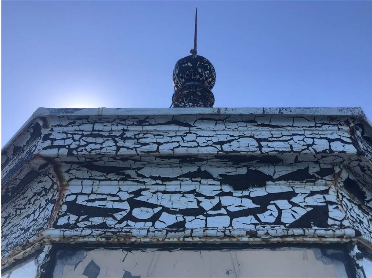
Photo 9. While degradation of the overpaint presents an image of vast deterioration, the underlying structure and surface conditions are sound. It looks far worse than it is. The ventilator ball and lightning protection system are intact and functioning; both are important contributors to the Lighthouse's well-being.
