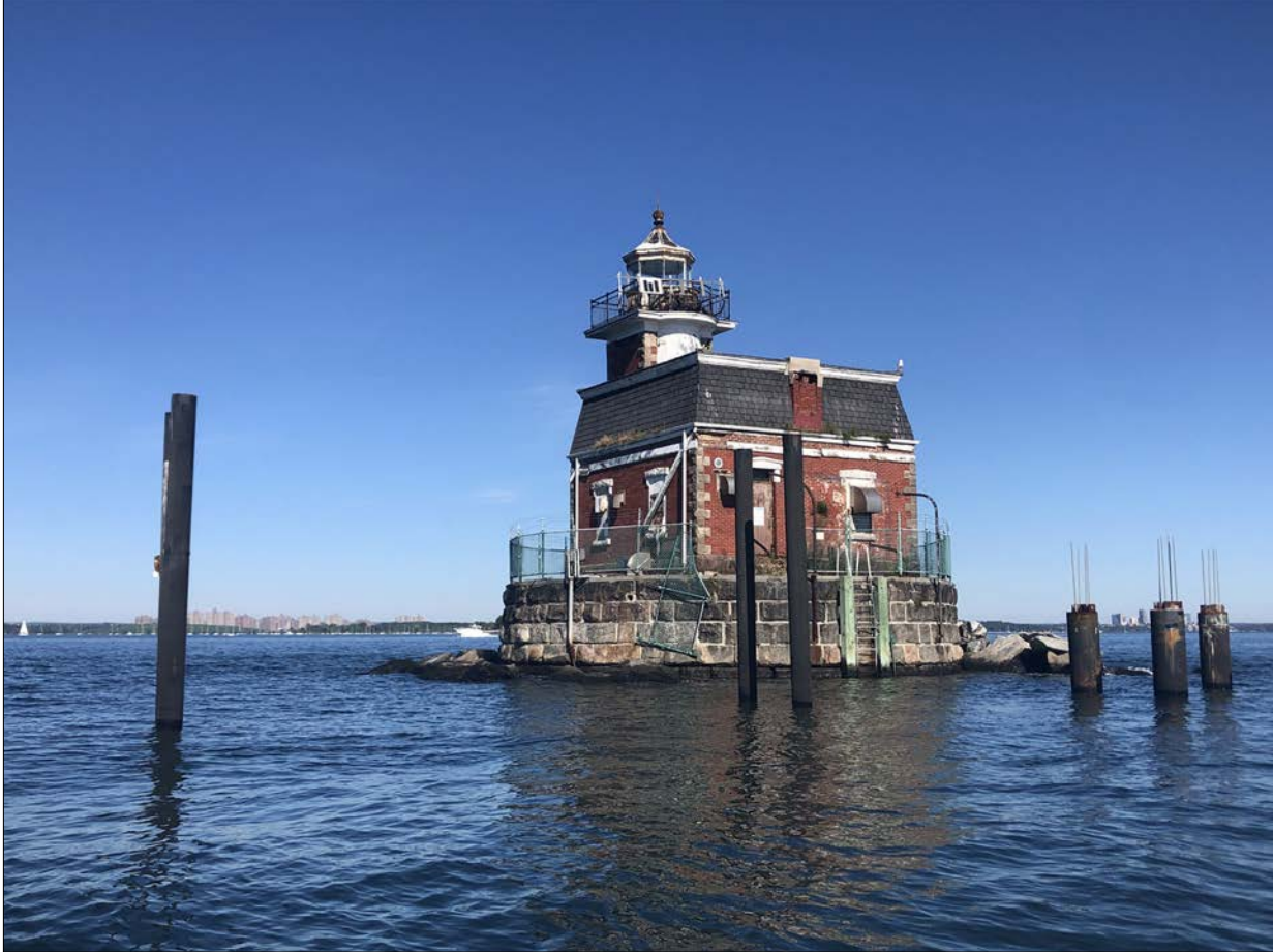
Photo 1. View of the approach to Stepping Stones Lighthouse, looking NE. Steel piles represent the initiation of a project to create a landing facility and gangway, which would simplify access for stabilization, restoration, ongoing operations & maintenance, as well as programmed visitation. Completion of the landing facility is an important and integral step in the ongoing stewardship of this historic Lighthouse.
