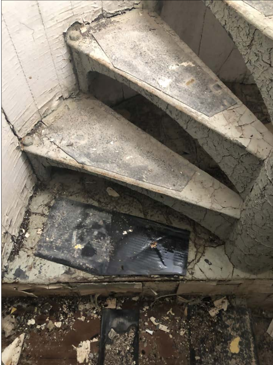
Photo 12. Accumulated water within Lantern dome liner is continuously dripping on Lantern stairs & flooring, affecting Service Level ceiling below.
